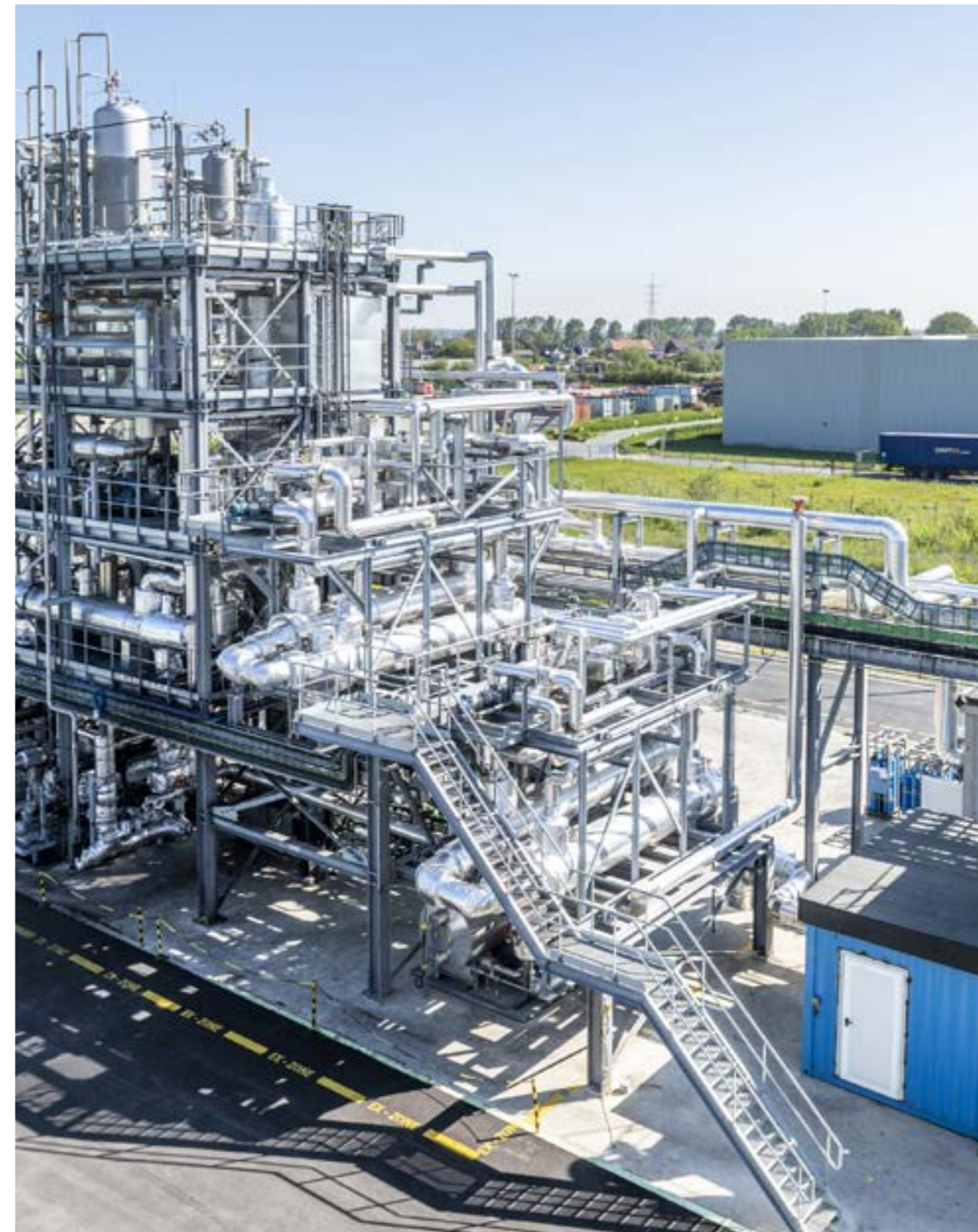
Renasci chemical recycling plant in Oostende. Bron Foto © Renasci / Borealis. www.sustainableplastics.com/news/borealis-signs-exclusive-agreement-secure-chemically-recycled-feedstock-supply
