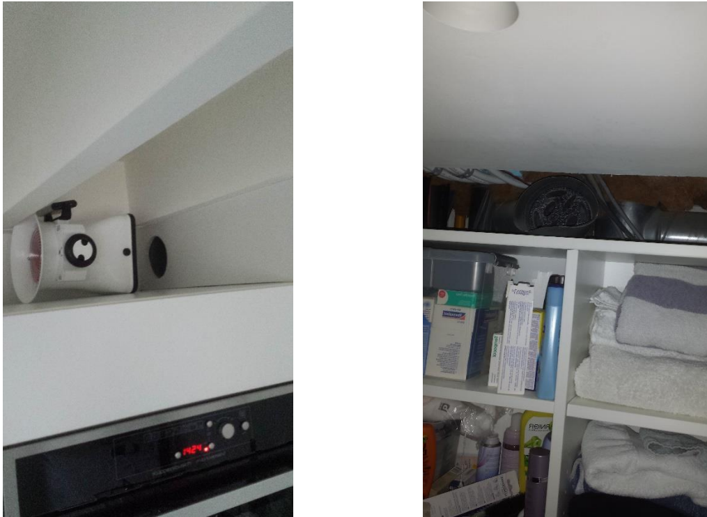
Figure 10: Sometimes the supply or exhaust outlet was difficult to access, leading to errors in the measurement of the air flow rate.
